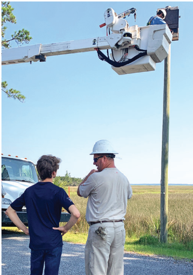
Richmond Hill Boy Scout Randall Singhas talks with Coastal Electric Cooperative Line Supervisor Clint Durrence as Lineman Hunter Hawkins installs bat boxes for Singhas' Eagle Scout project.
