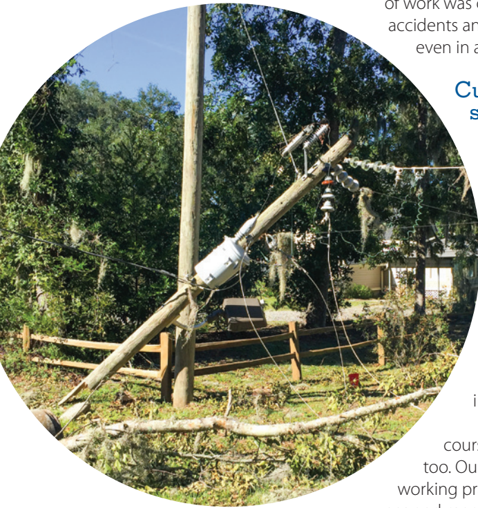
Equipment lies in a tangled mess in the Lake George community Oct. 11, compliments of Hurricane Matthew. It took three Coastal Electric linemen and five outside crews two days to clean up and restore power to the area.
