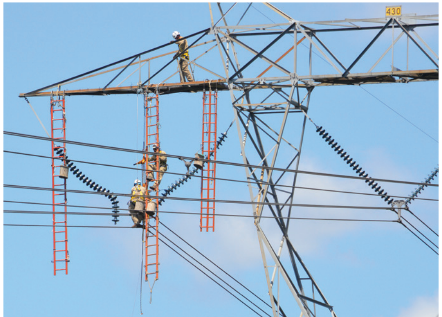
Linemen work from a helicopter on April 16 to replace porcelain insulators on the 500,000-volt transmission line that runs along Hwy. 17 in Richmond Hill.
